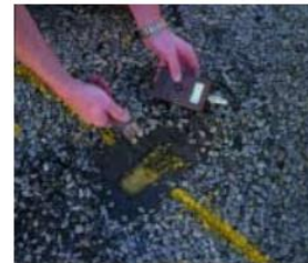
Moisture probe testing quickly confirms the presence of moisture.
