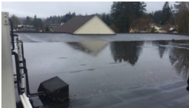
Plenty of drains, roof well maintained, but the low areas between the drains needed crickets to push water to drain.
