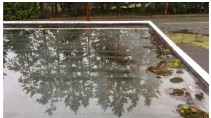
Ponding water due to a lack of maintenance and plugged drains clogged.
